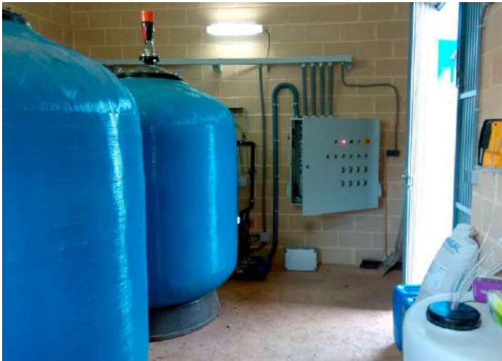
Figure 1: BIOBOX Nitrate Biofiltration Plant with 88 GPM Capacity
