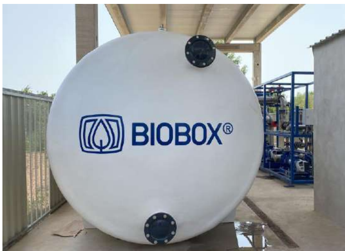
Figure 1: BIOBOX Nitrates Biofiltration Plant of 528 GPM (Recirculation, supply 880 GPM) / 120 m 3 /h (Recirculation, 200 m 3 /h)
