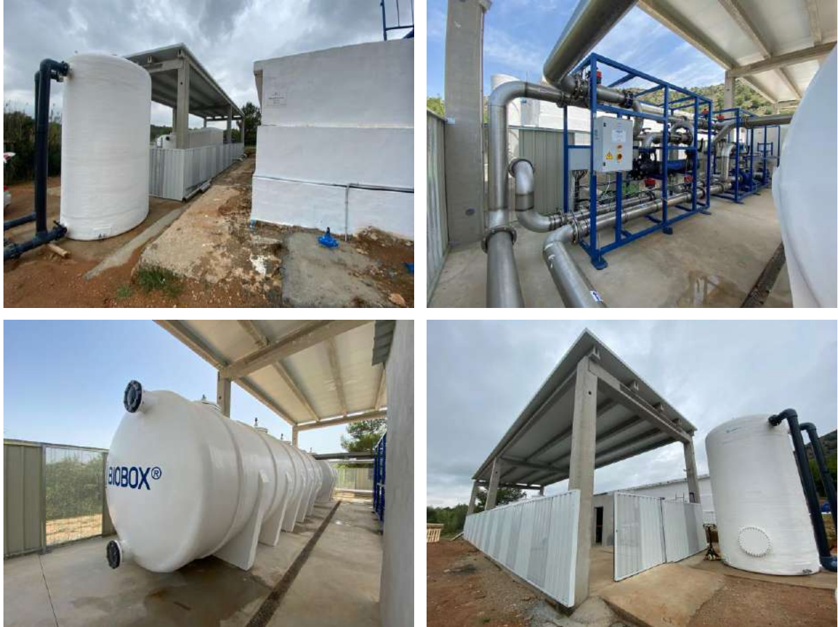
Figure 2: Interior/Exterior Images of the BIOBOX Nitrate Biofiltration Plant of 528 GPM (Recirculation, supply 880 GPM) / 120 m 3 /h (Recirculation, 200 m 3 /h)
