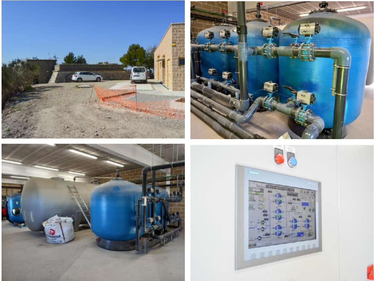
Figure 2: Interior / exterior images of the BIOBOX Nitrates Biofiltration Plant with 88 GPM capacity / 20m 3 /h
