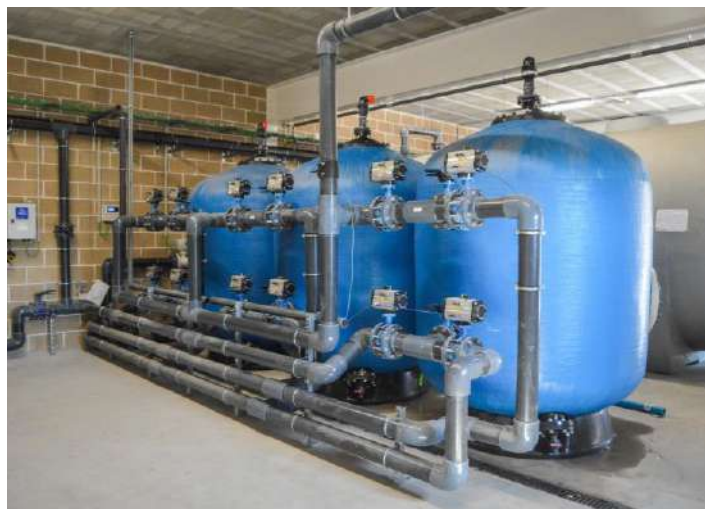
Figure 1: BIOBOX Nitrate Biofiltration Plant of 88 GPM / 20m 3 /h
