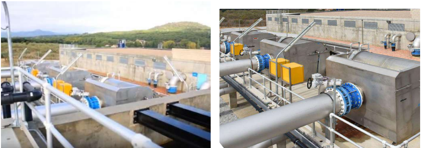
Figure 2: Images of the Pelayos de la Presa WTP; Canal de Isabel II
