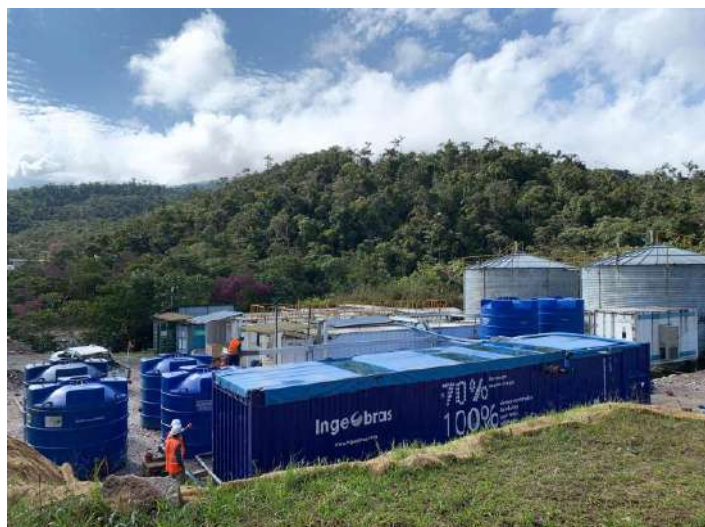
Figure 1: BIOBOX Plant of 30 GPM, which is equivalent to 7 m³/h.
